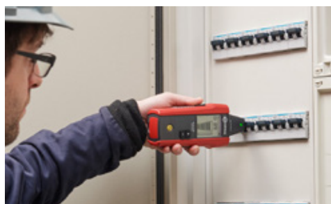
Identify the single correct breaker
